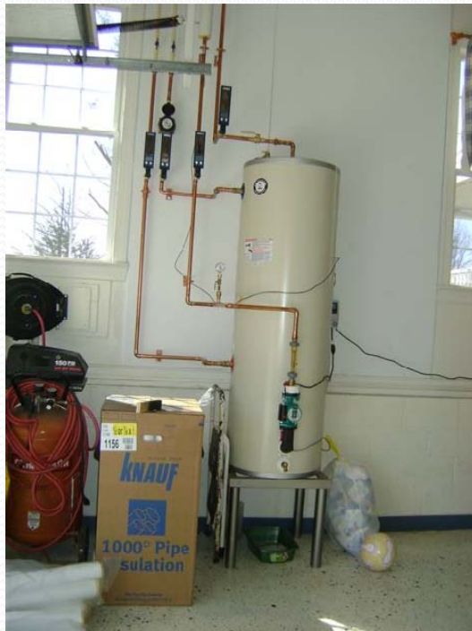
Solar Thermal Drain Back Tank & Piping
